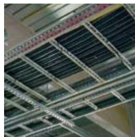
HEAVY DUTY PERFORMANCE WITH CABLE LADDERS
